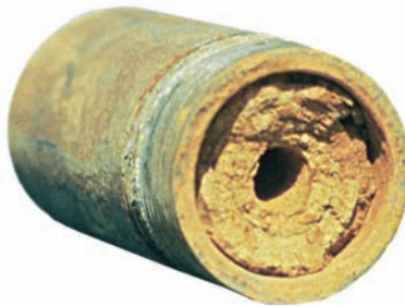
Hard water deposits in pipes
