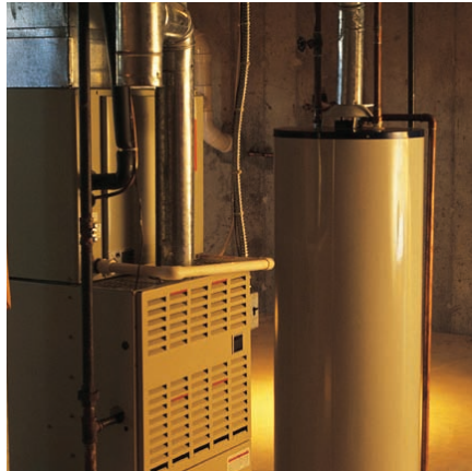
Poor water quality can damage your plumbing and your appliances
